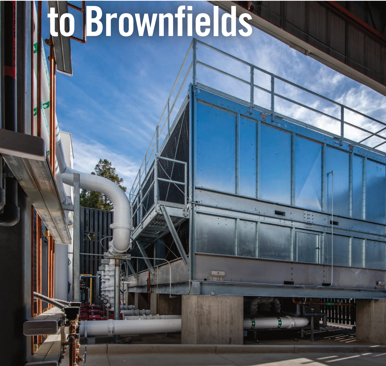
A chiller tower for a data center.
