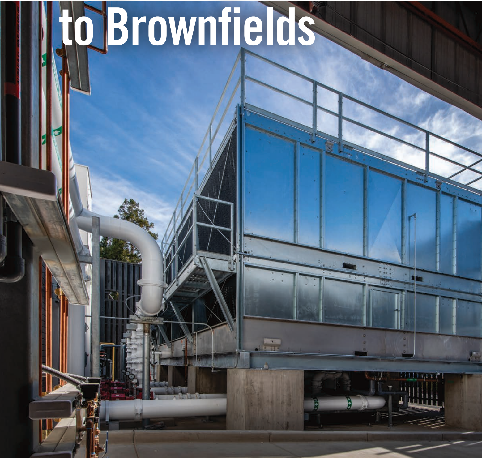
A chiller tower for a data center.
