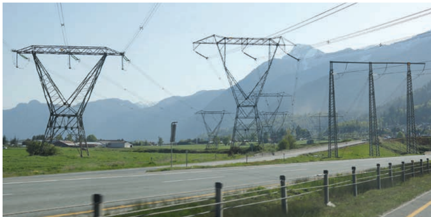
Transmission towers near the Trans-Canada Highway in British Columbia's Fraser Valley.
