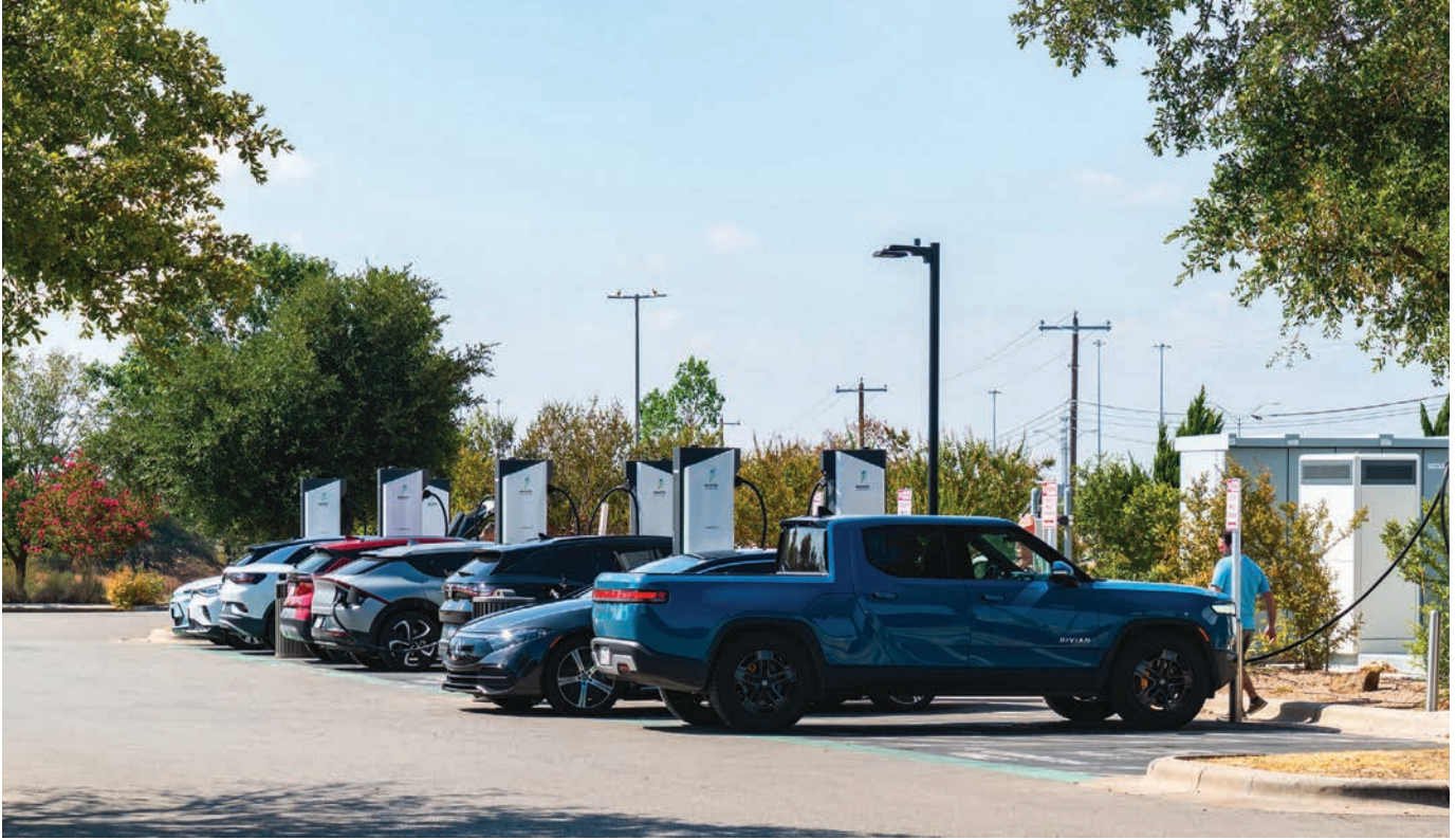
The process for getting an EV charging station up and running can take as long as two years.
