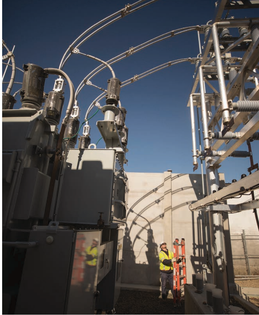
Power transmission upgrades can be a challenge on par with generation capacity in some markets.
